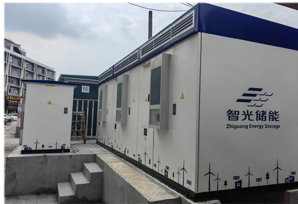
Modular LV ESS System
